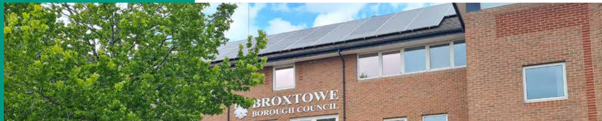
Image 2: Solar PV on the main Council offices at Foster Avenue - Beeston
